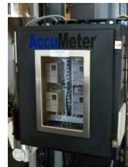
Motor drive panel
