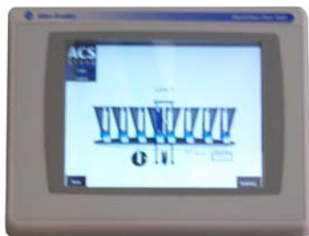
Allen-Bradley control system interface
